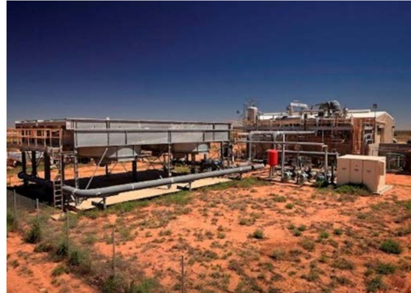
Habanero Pilot Plant, Cooper Basin (Australia)
