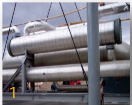
The Beowawe Power Plant , a low-temperature, binary cycle plant, uses waste heat from an existing geothermal plant at the facility, which has added 1.8 MW to the existing plant's nameplate capacity of approximately 17.7 MW. The project was funded in part by the geothermal Technologies Office under the American Recovery and Reinvestment Act. Photo courtesy of Terra-Gen
