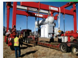
The Rocky Mountain Oilfield Testing Center (RMOTC) Relocation Project is designed to reduce the risks associated with co-production by operating binary units in commercial oil and/or gas fields. Technical site data will be collected to significantly reduce cost and performance uncertainties and lower the barrier for market uptake.
