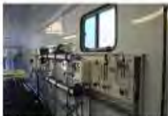
Interior of unit, set up for membrane modules
