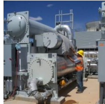
ORC Heat to Power
