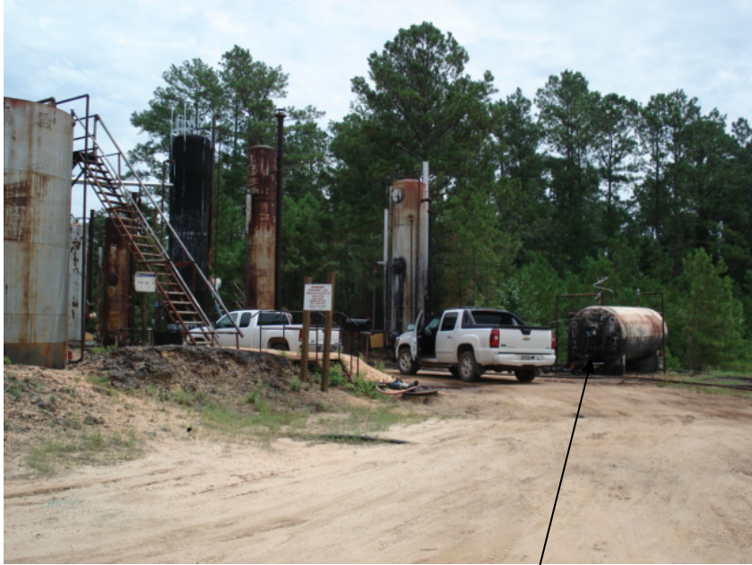
#22 Battery. Production Separator
