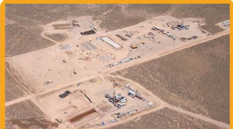
A July 2008 aerial view of the site shows two drilling rigs, the concrete foundation for the cooling towers, and foundation preparation for the generator array.
