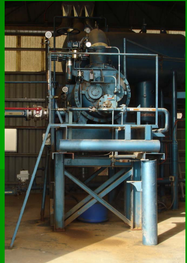
Birdsville, 80 kWe net ,ORC power plant
