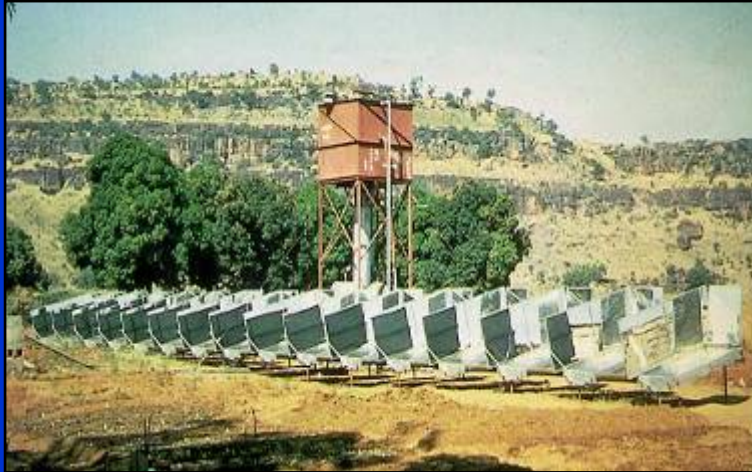
Solar Water Pump System, Mali
