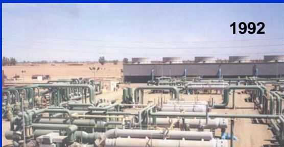
40 MW Heber Geothermal No. 2 Binary Power Plant, California,
