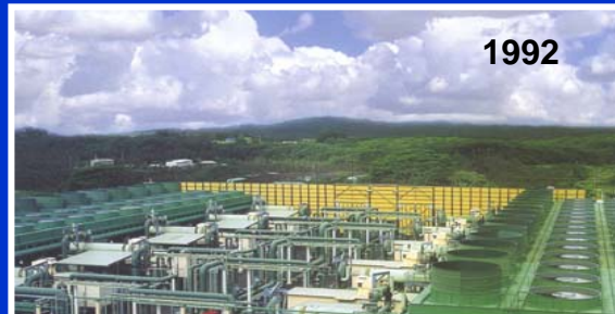
30 MW Puna Combined Geothermal Power Plant, Hawaii
