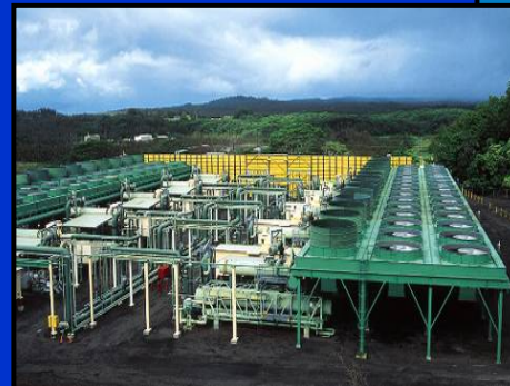
30 MW Puna Geothermal Power Plant, Hawaii
