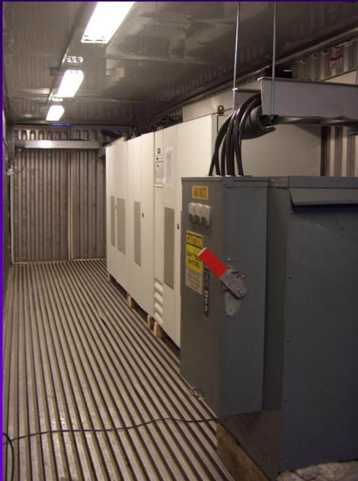
UPS System (MGE)
