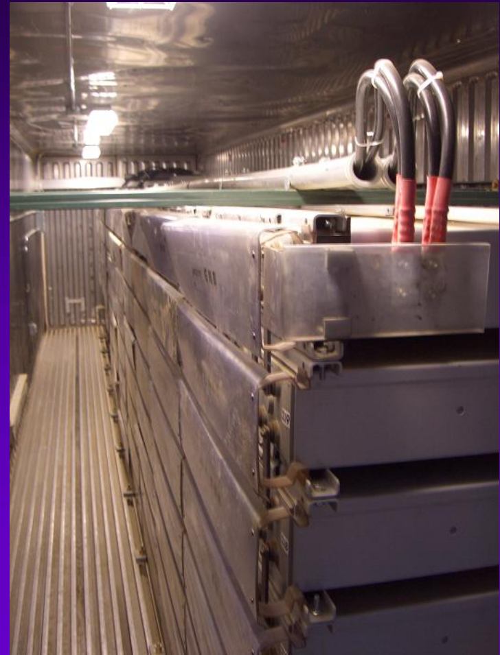
Batteries 3MW Total
