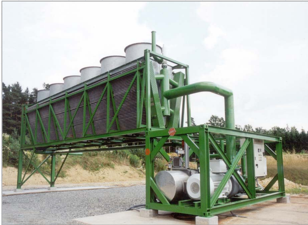
Series 250 Containerized ORMAT Energy Converter Power Unit at Rogner Hotel & Spa, Bad Blumau, Austria
