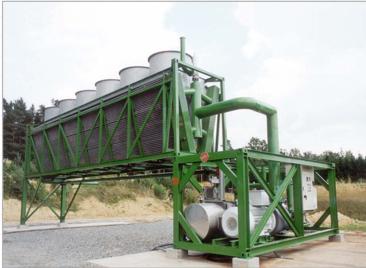
Series 250 Containerized ORMAT Energy Converter Power Unit at Rogner Hotel & Spa, Bad Blumau, Austria
