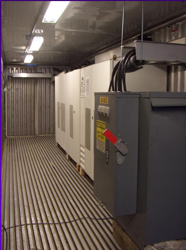
UPS System (MGE)
