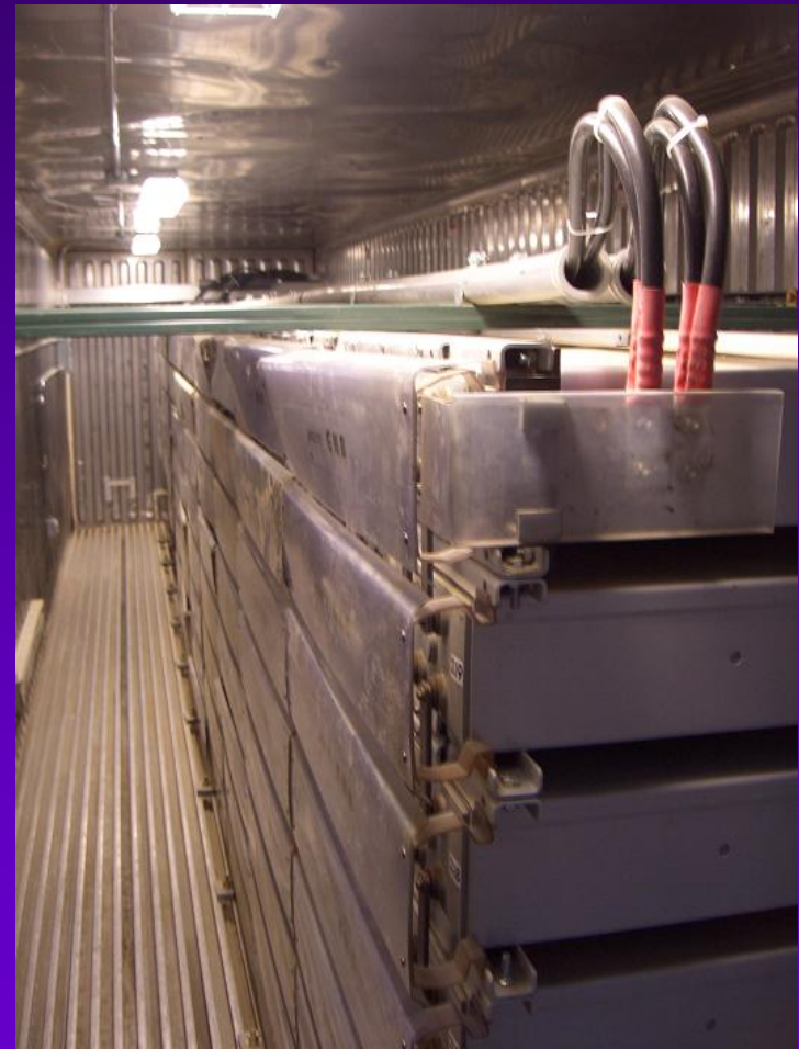
Batteries 3MW Total
