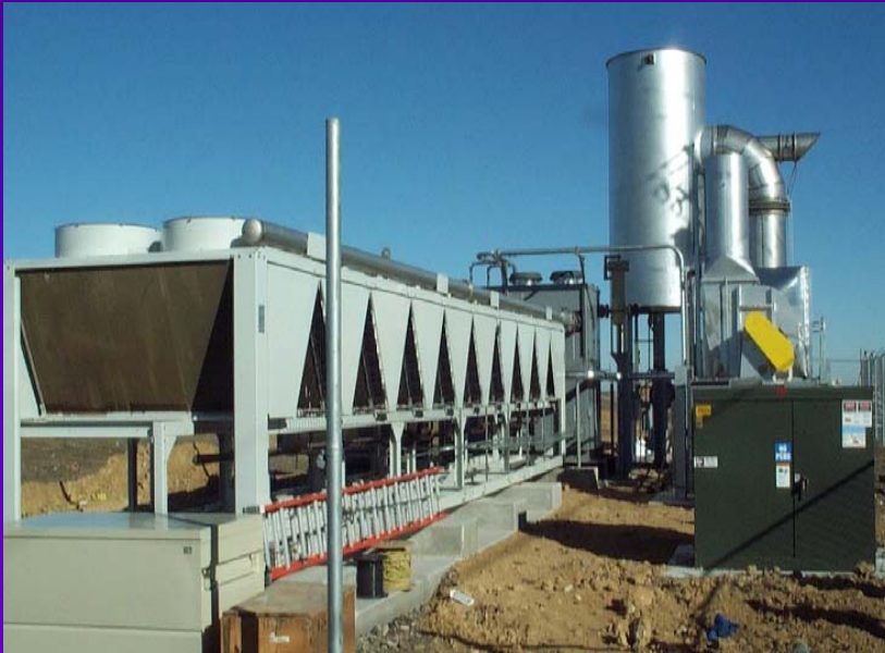
PureCycle 200 Operating off Landfill Flare in Austin, TX
