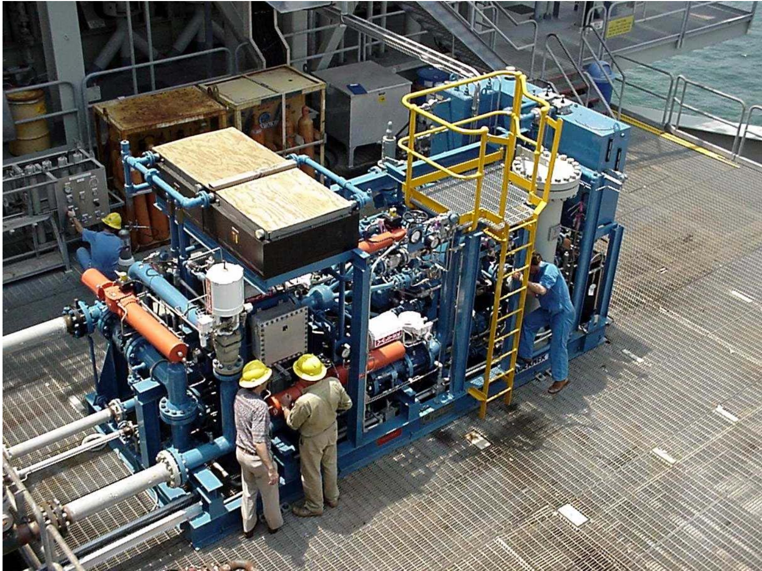
Two-Phase Separating Turbine on Ram-Powell Platform, after Dresser-Rand
