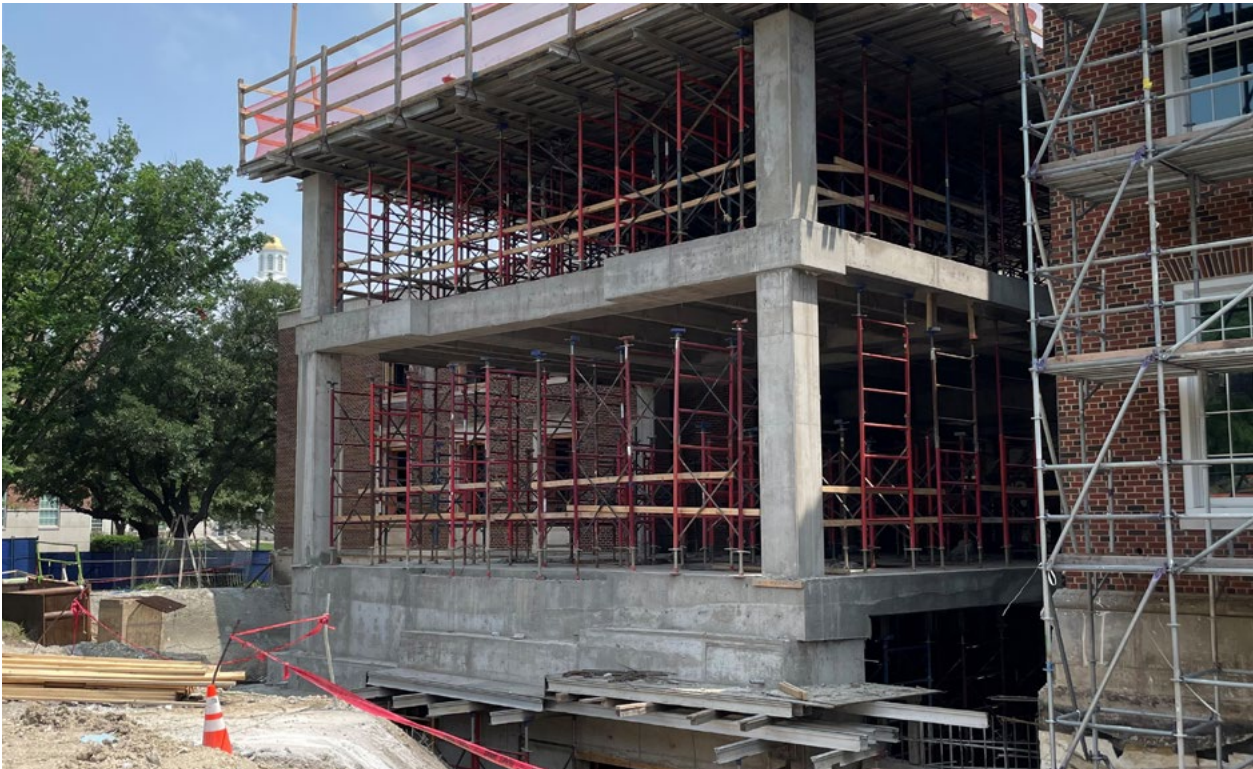
Shaddock Hall, on the northeast side of the complex, has made substantial progress from March to June.
