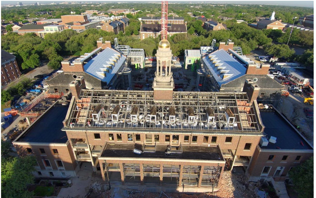
The Fincher Building roof is down to the studs in April. The new terrace is seen from above in this east-facing view.
