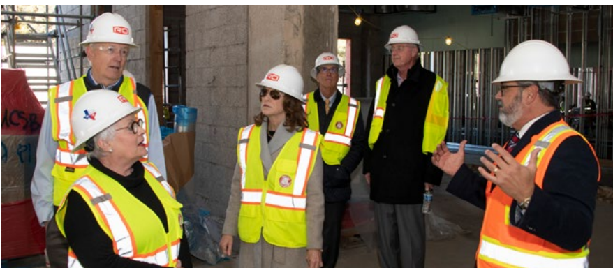
SMU Associate Vice President of Facilities Planning and Management and University Architect Michael Molina (far right) answers questions on the January building tour. Also pictured (left to right): Tucker Bridwell, Carolyn Miller, Gina Myers, Dean Matthew Myers and David Miller.
