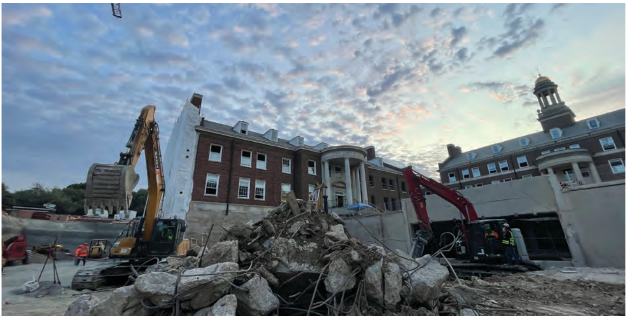
The view of the Maguire Building from what used to be the Bishop Boulevard-side exterior steps (that led to the Business Library), reduced to rubble in August.
