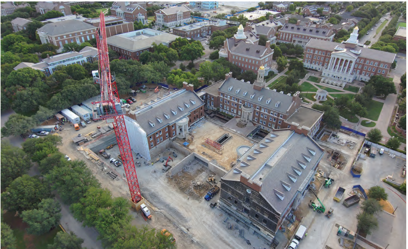
An aerial view of the renovation and expansion site on July 29, 11 weeks after the beginning of construction.
