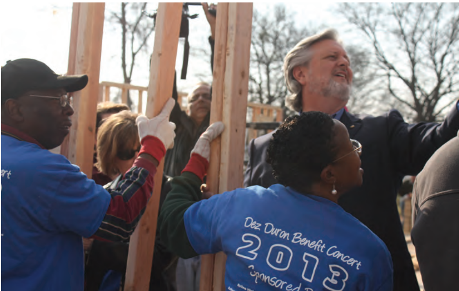
Barry Hughes (upper right) looks upward as a frame wall is secured
